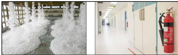
Figure 8. Foam Extinguishing System and Fire Extinguishing Devices
