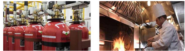
Figure 10. Fm 200 Extinguishing Systems and Hood Extinguishing System
